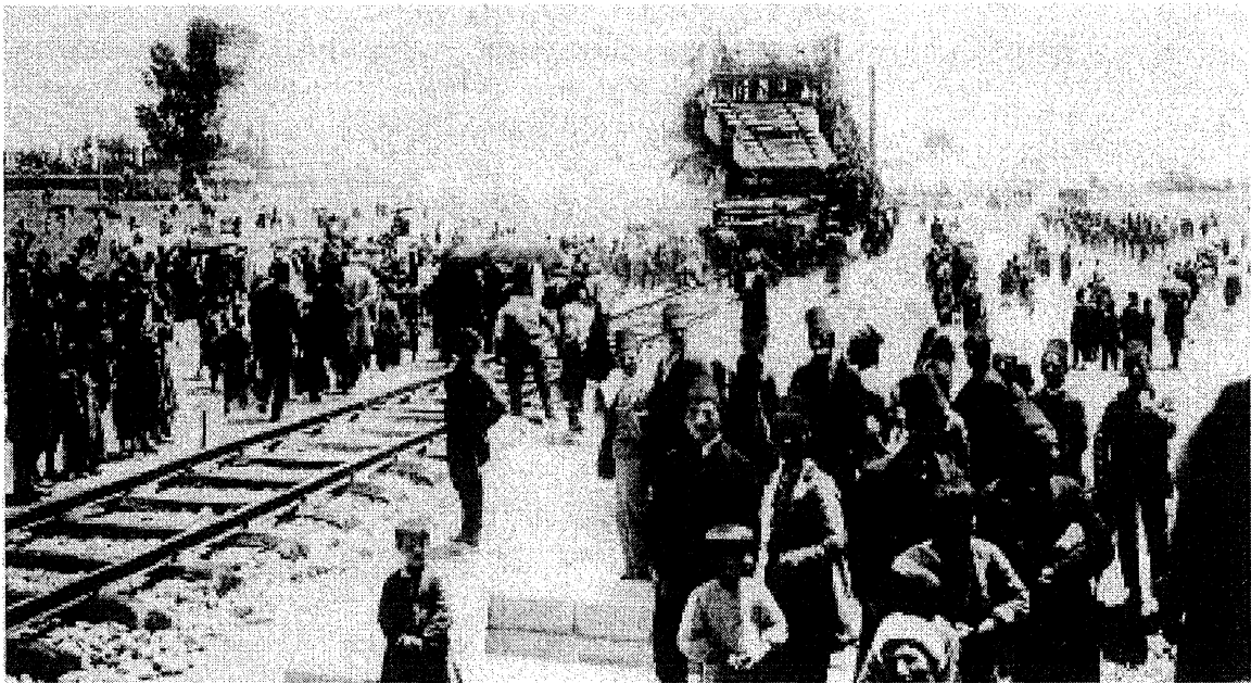
Construction work on the Eskişehir-Konya line of the Anatolian Railway Source: Pohl, Vom Stambul nach Bagdad , p. 45
