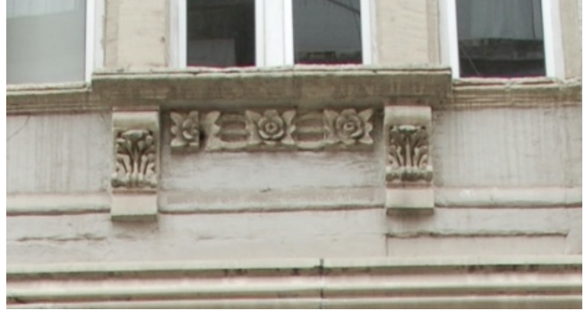
Figure 132: Unknown Architect, Sureya Bey Apartment – rose motif detail (under the windows) , Meşrutiyet Boulevard No:14, early 1900s. Photo: Merve Uca
