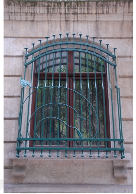
Figure 105: Unknown Architect, Rassam Apartment – window detail (ground floor), Çukurcuma, 1905. Photo: Merve Uca
