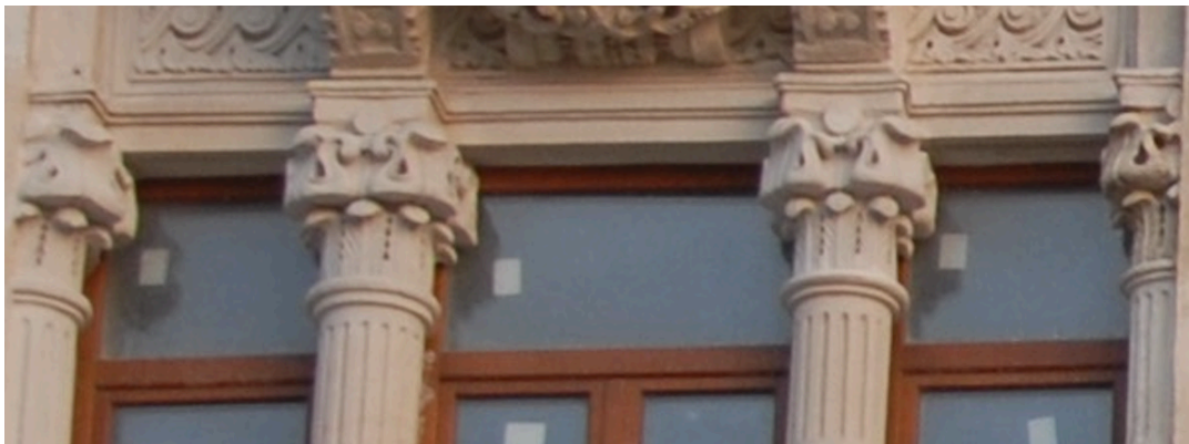
Figure 59: Konstantinos Kyriakides and Alexandre Néocosmos Yenidunia, Freige Apartment – detail from main façade, Şişhane, late 1900s. Photo: Merve Uca
