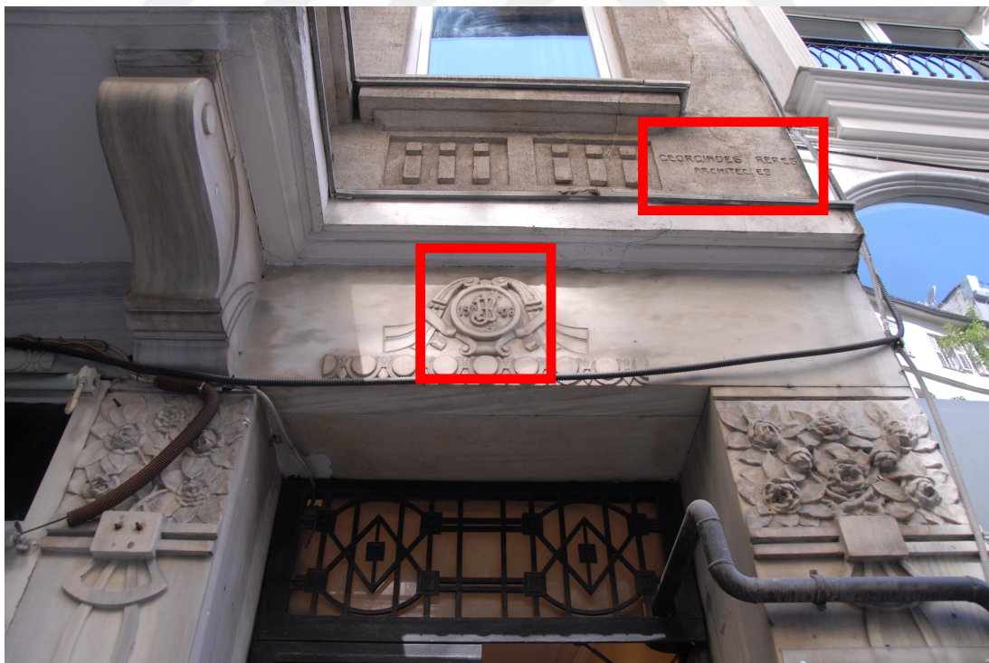
Figure 70: Dimosthenis & Stefanos Georgiadis, Çağdaş Apartment – detail from the entrance door, Meşrutiyet Boulevard n. 68, Istanbul, 1906. Photo: Merve Uca
