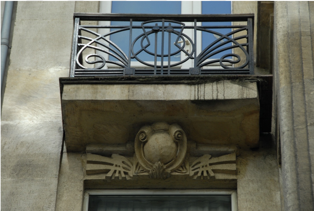
Figure 73: Dimosthenis & Stefanos Georgiadis, Çağdaş Apartment – balcony detail, Meşrutiyet Boulevard n. 68, İstanbul, 1906. Photo: Merve Uca
