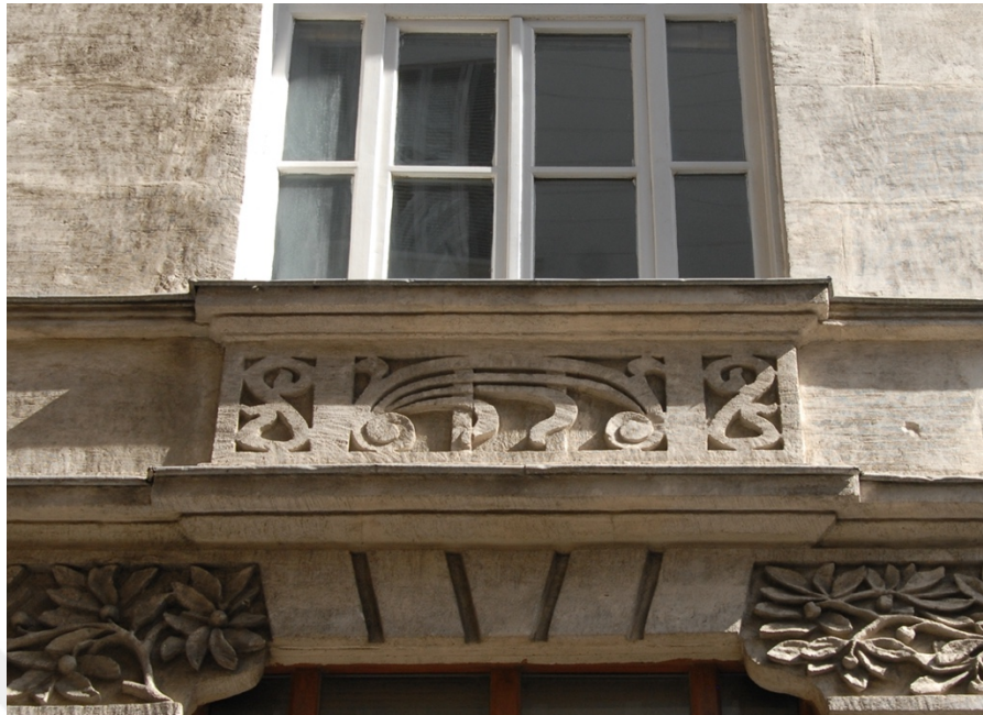
Figure 80: Dimosthenis & Stefanos Georgiadis, Abouaf Apartment – window detail, Şişhane, early 1900s. Photo: Merve Uca
