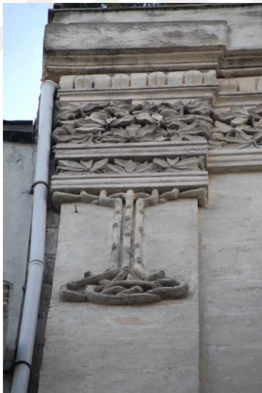
Figure 115: Unknown Architect, Atlas Apartment – detail , Asmalı Mescit, early 1900s. Photo: Merve Uca
