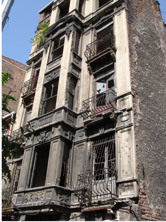
Fig. 12 A decaying apartment building in Cihangir, photograph taken by the author, 2006
