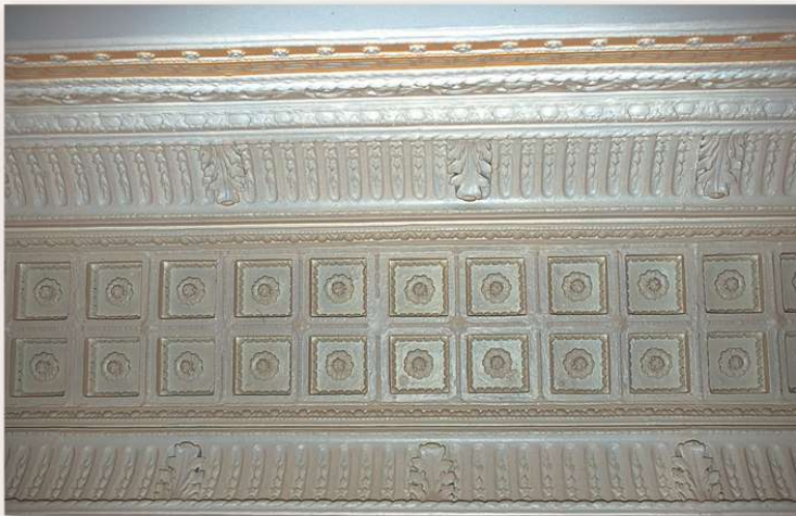
The ceiling is alternatively made of caissons punctuated by rosettes in some parts and panellings in other.
